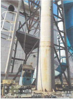
磨背锥废气排气筒
